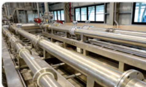
Piping system II (Maximum diameter is 300mm)
