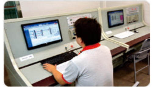
Control room & Graphical HMI
